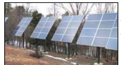
Solar panels at Lifebridge Sanctuary in Rosendale Photo by Patty Matteson
